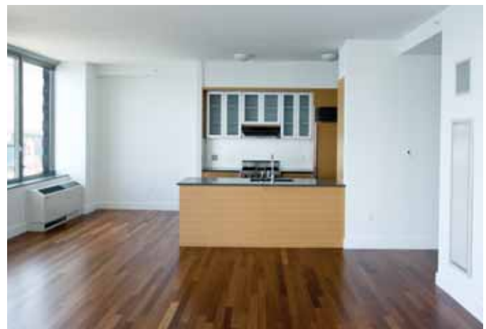
The kitchen of a Tower condo features a ClimateMaster console unit and a vertical unit in the living area
