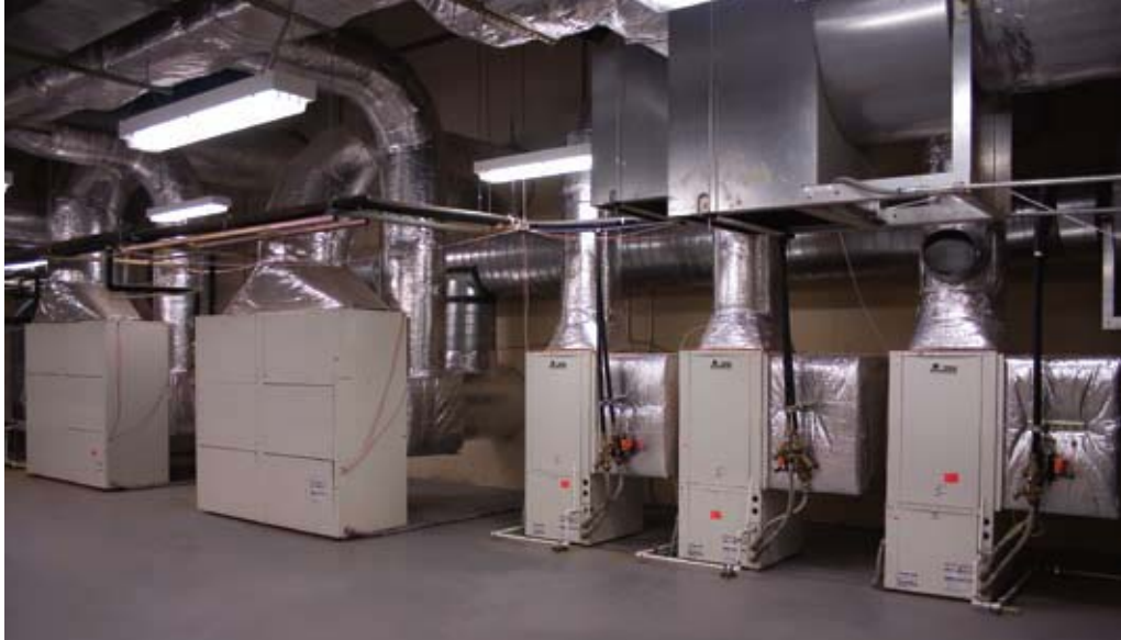
ClimateMaster heat pumps at work in Western Heights Middle School
