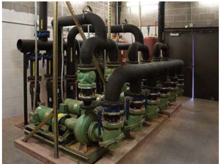
The pump room at Western Heights Middle School
