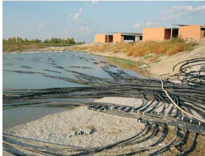
Fused header assemblies for the pond loop system.
